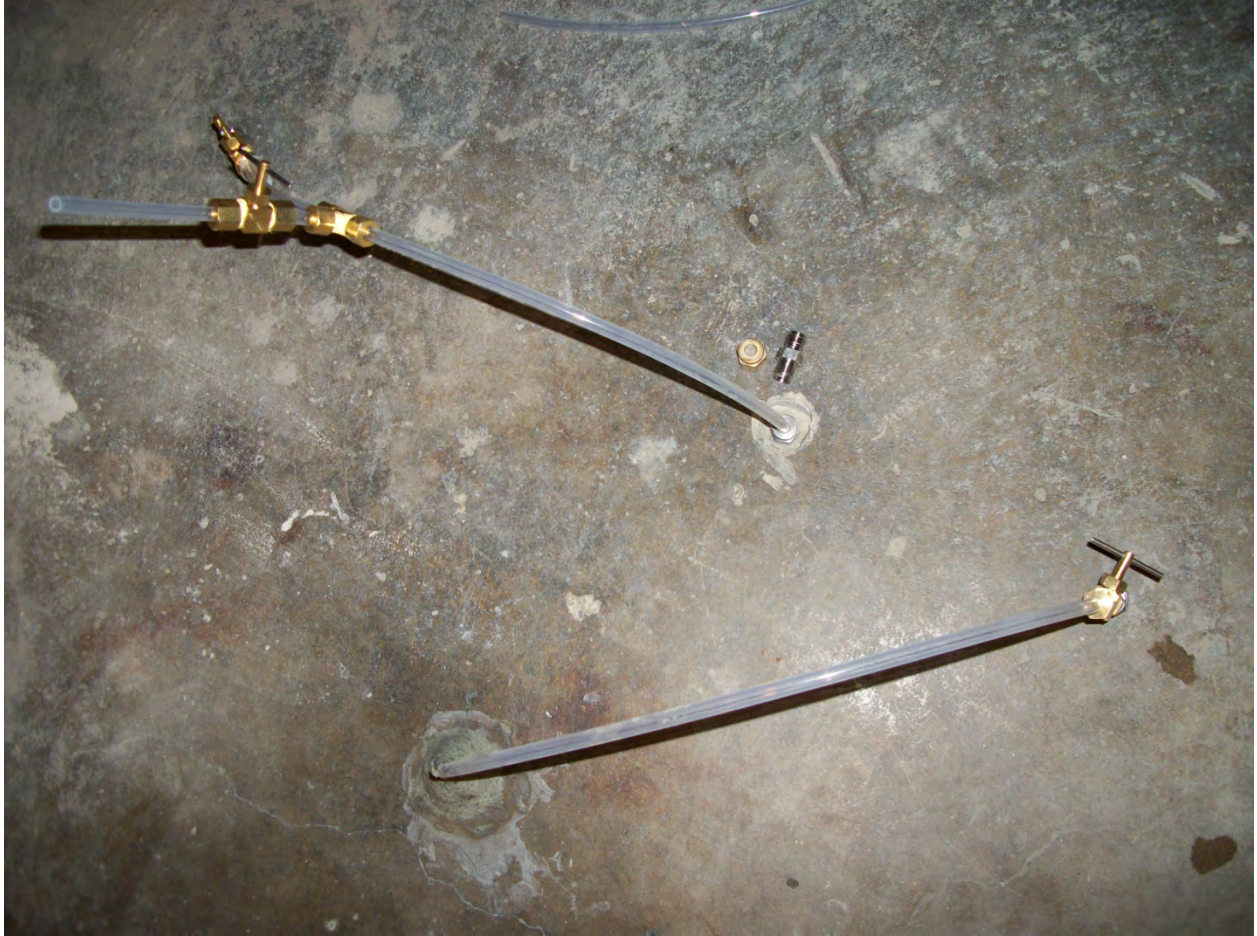
Typical Port Construction Before Sampling, One Temporary port shown at lower end of picture and one Permanent port shown in the middle of the frame
