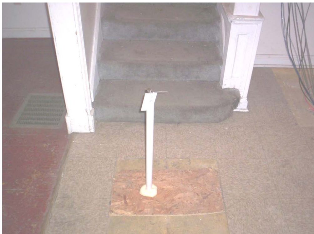
Figure 3-24. Monitoring well MW-3, installed in the basement and completed on the first floor.
