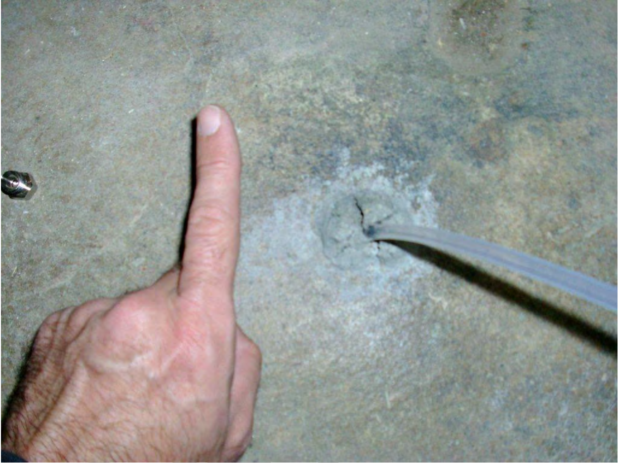
Temp Port 1 close up
