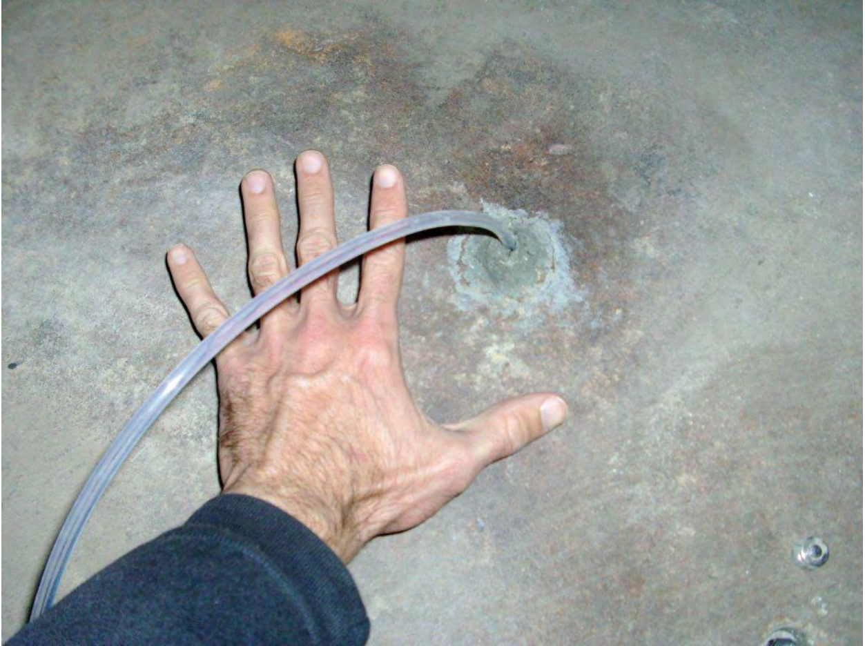
Temp Port 5 close up
