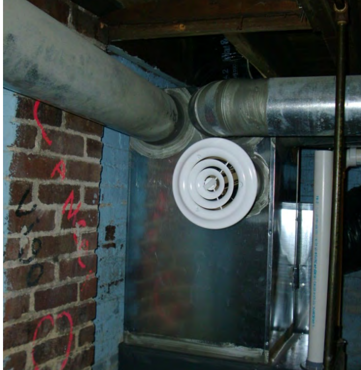
Figure 3-11. Basement supply register in newly installed HVAC system.
