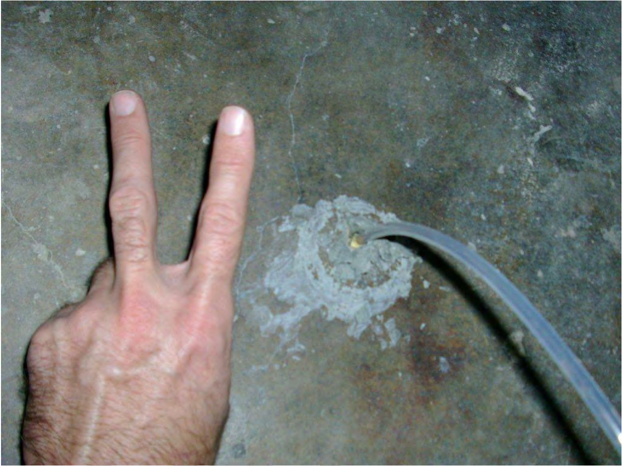
Temp Port 2 close up
