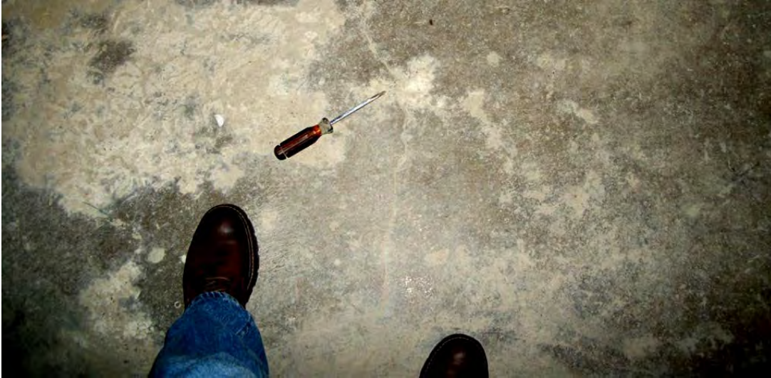
Figure 3-14. Floor cracks in 422 basement, central area, contrast enhanced.
