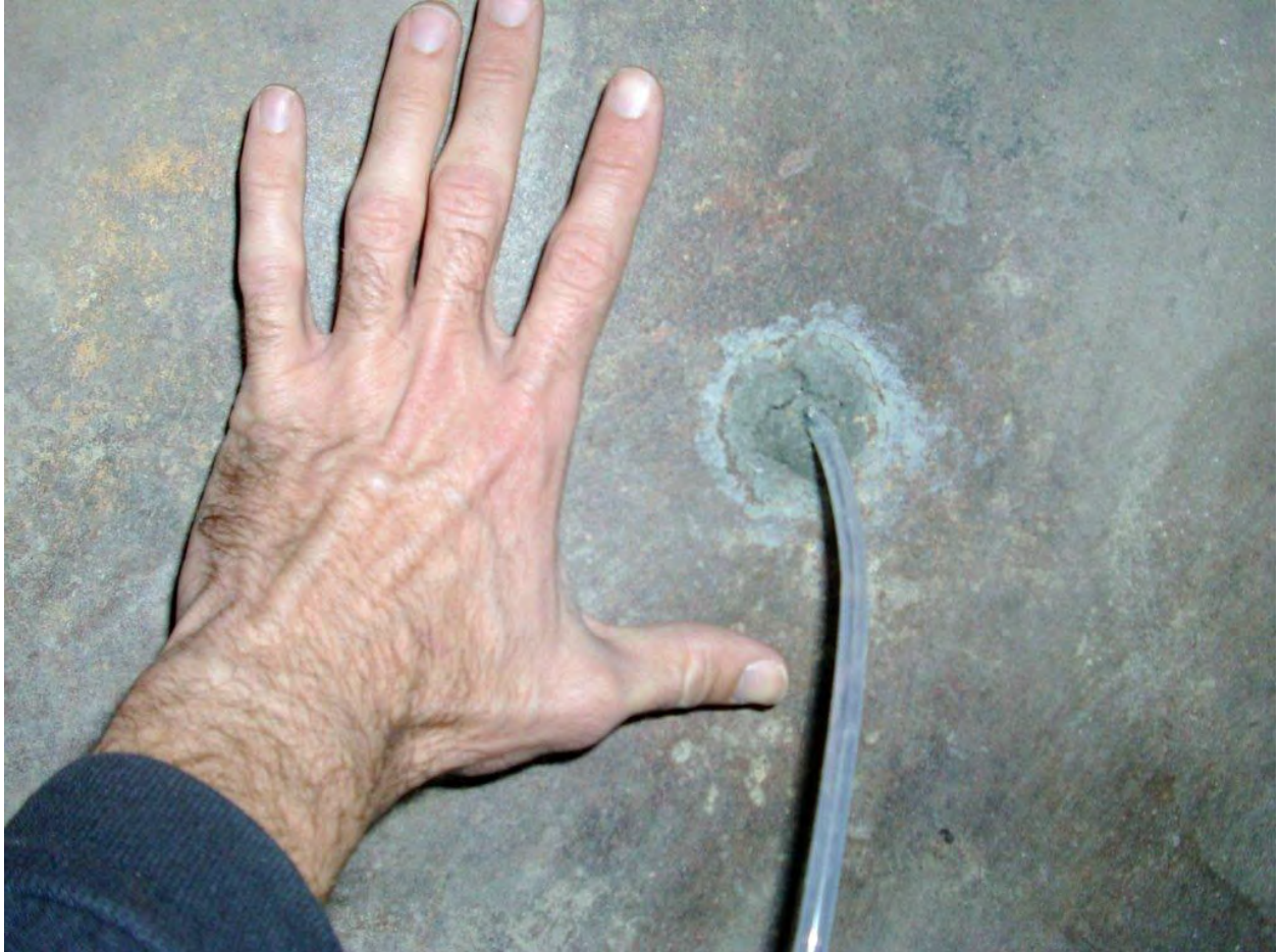
Port 5 additional close up
