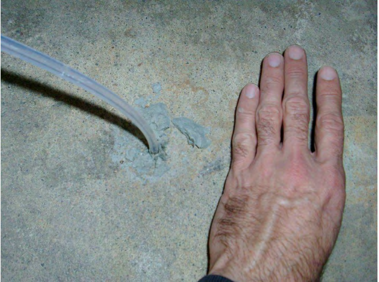
Temp Port 4 close up
