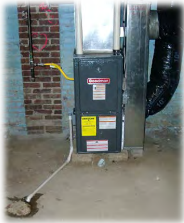
Figure 3-13. Gas-fired forced hot air HVAC system installed in 422.
