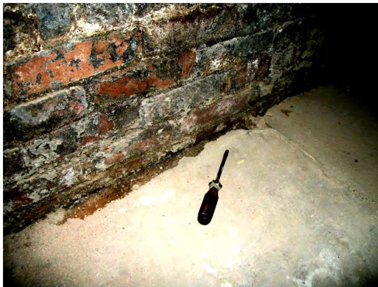
Figure 3-15. Weathered cement in walls and floor cracks in 422, contrast enhanced.
