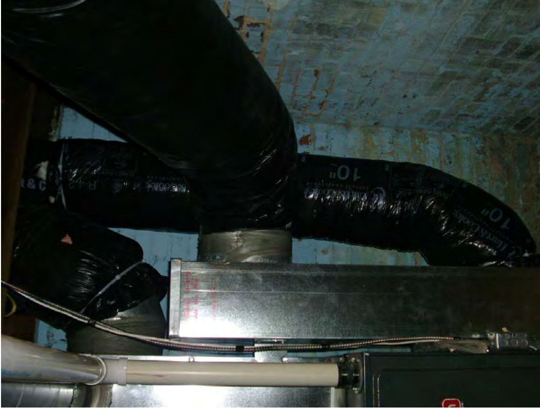
Figure 3-12. Common returns from first and second floors in newly installed HVAC system.
