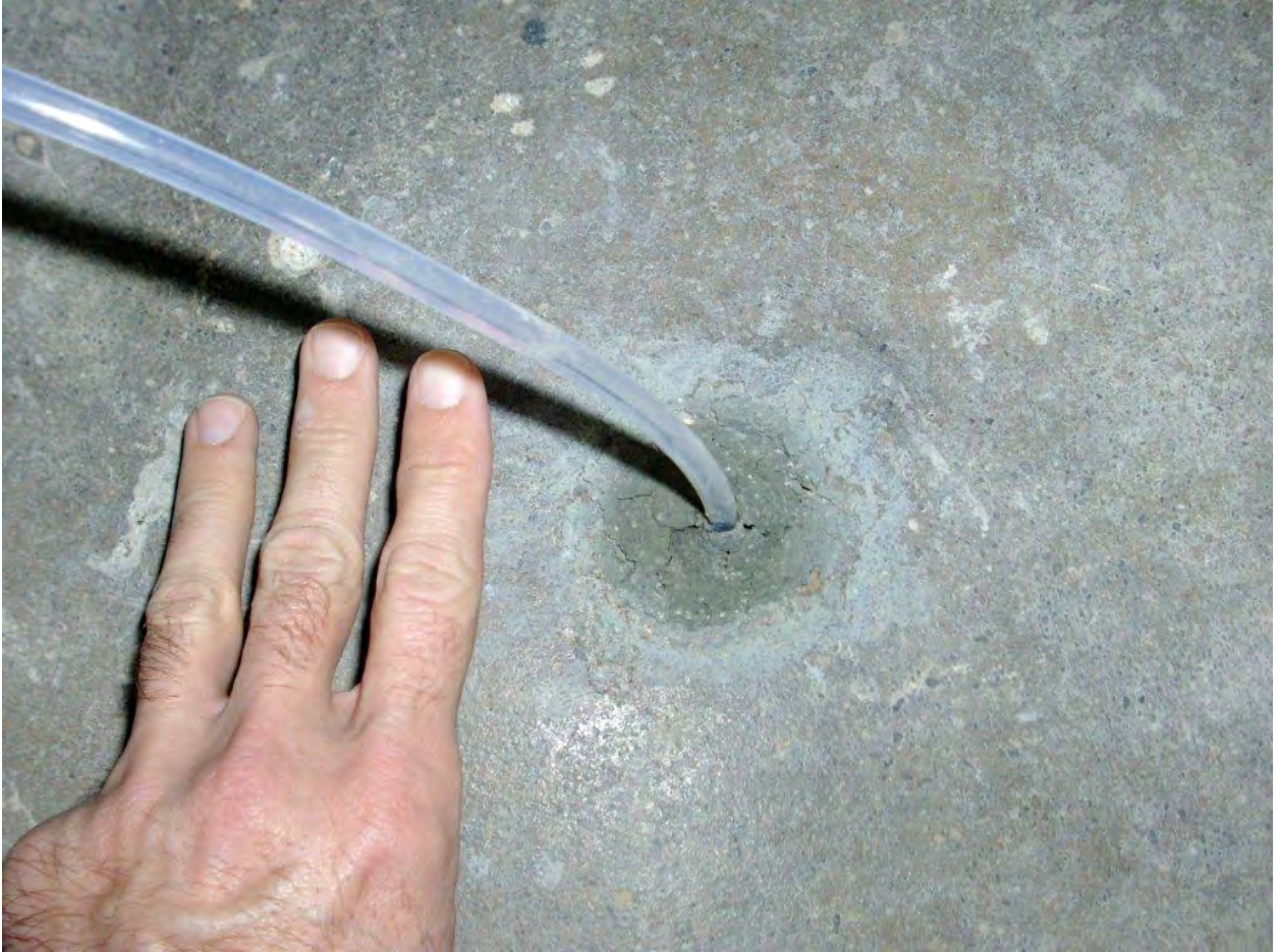
Temp Port 3 close up
