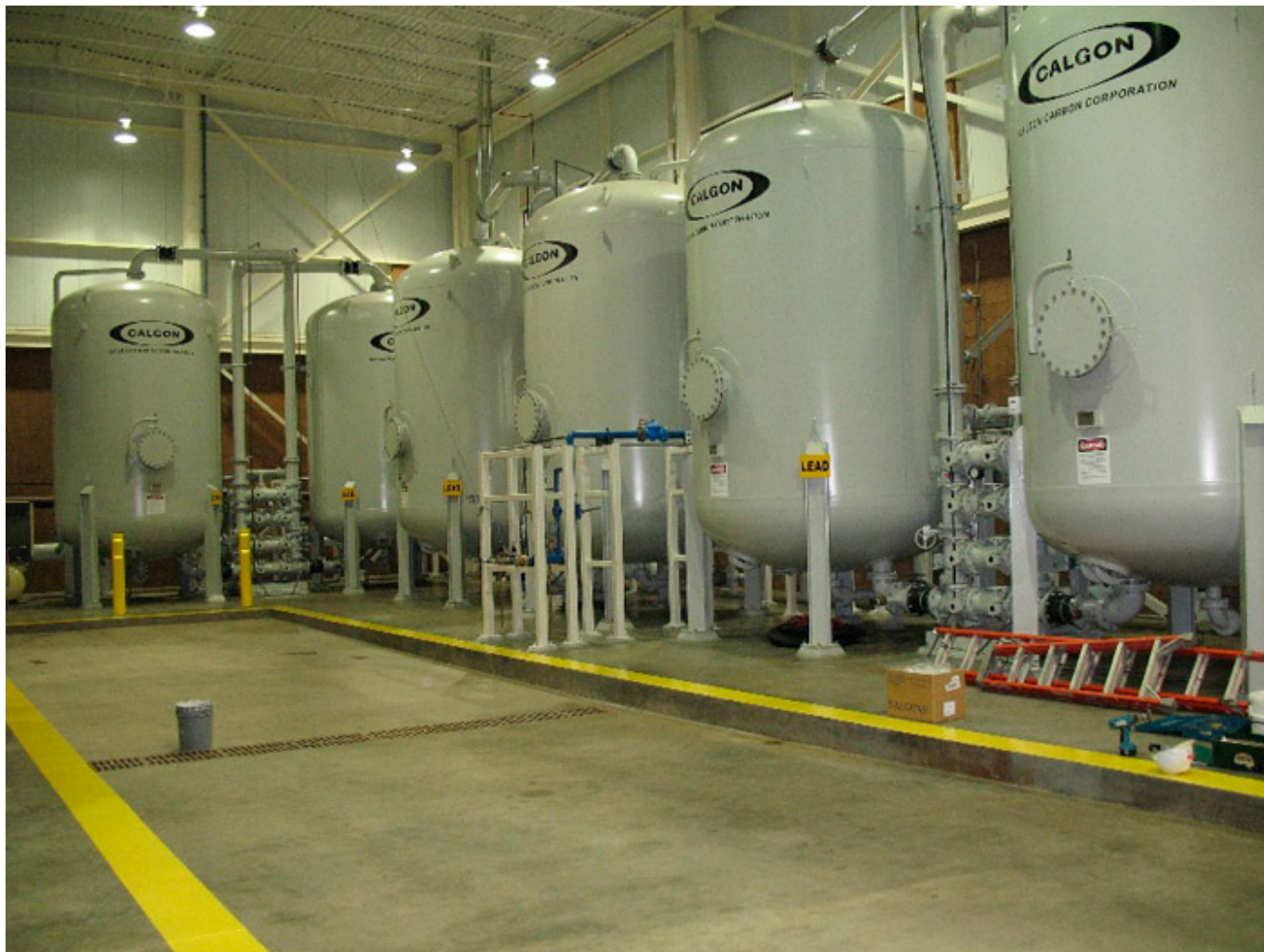
Figure 15-6. GAC treatment system, Oakdale, MN.
