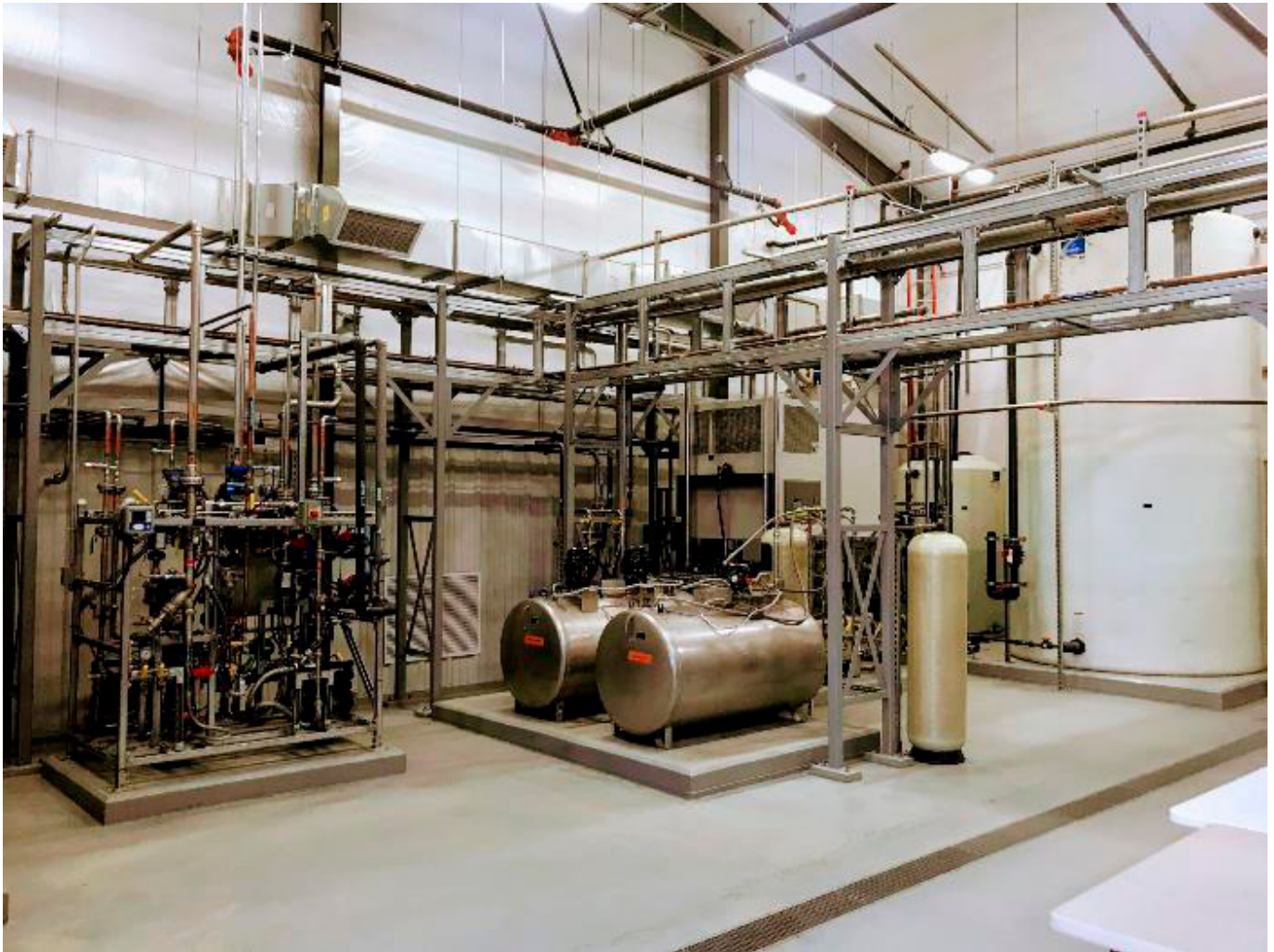
Figure 15-14. Resin regeneration system.
